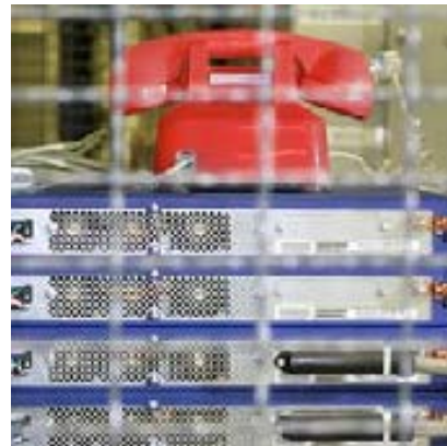
Overloaded lines and infrastructure
