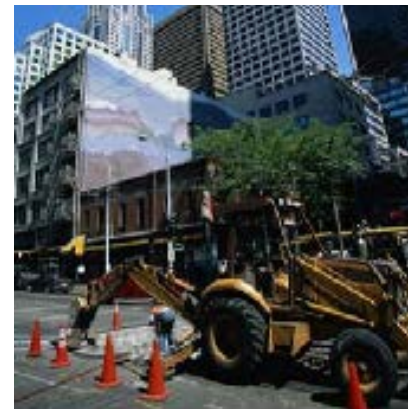
Cut cables and power
