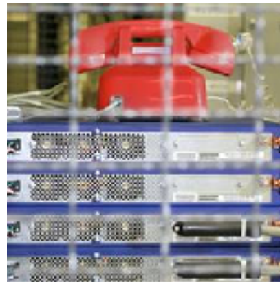
Overloaded lines and infrastructure
