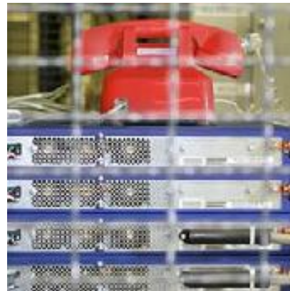
Overloaded lines and infrastructure
