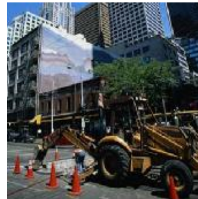
Cut cables and power
